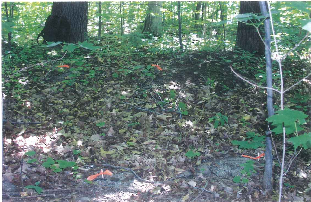
Fig. 7. Orange flag tape in 4 places marks where the geotextile was exposed. Photo taken June 18, 2002, looking roughly east.
