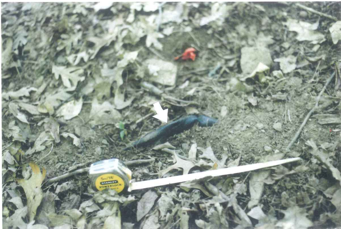
Fig. 6. At the white arrow is an example of an exposed piece of geotextile, approx. 8 in. long (tape is set at approx. 1 ft.) and located on the west edge of the stabilized pit. Photo taken Aug. 6, 2001.
